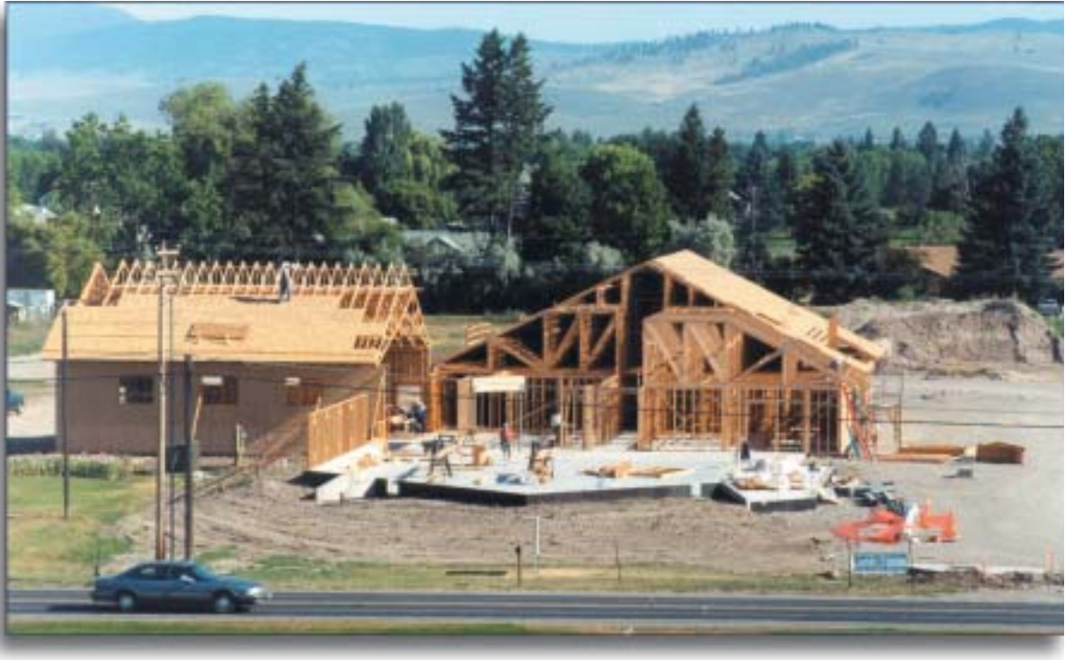
A view of the construction from the roof of Community Hospital on July 23, 1999
