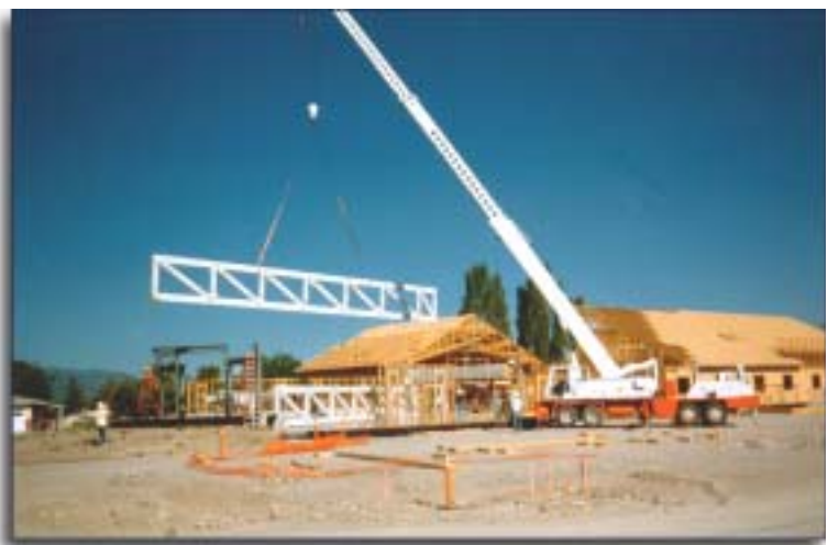
A crane with a 100 foot boom is shown lifting into place one of the two interior 6-ton beams.
