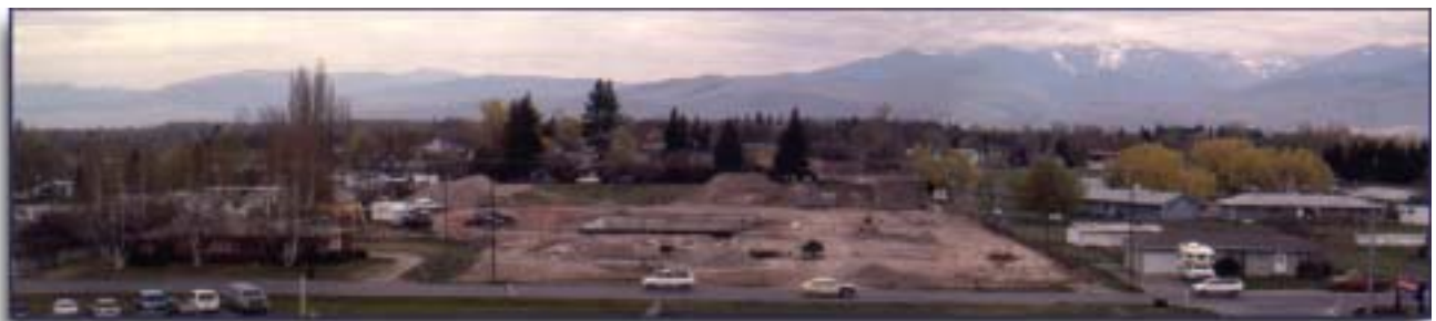
A view of the construction as seen from the roof of Community Hospital - April, 1999.
