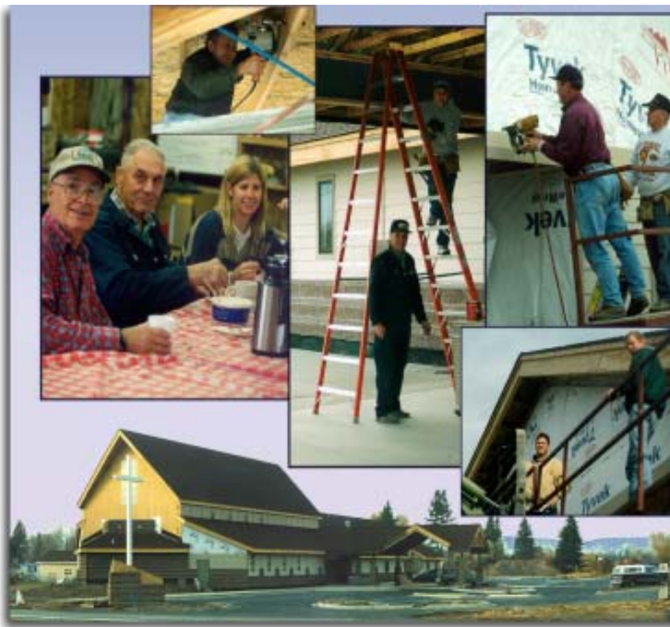
A view of the progress on the new church and some of the volunteer workers - November 11, 1999.
